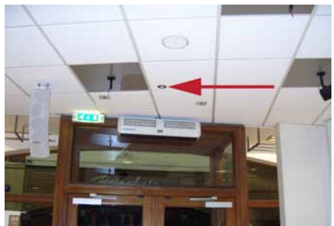
OptoCount installation in the BOSE shop, Portsmouth, UK.
